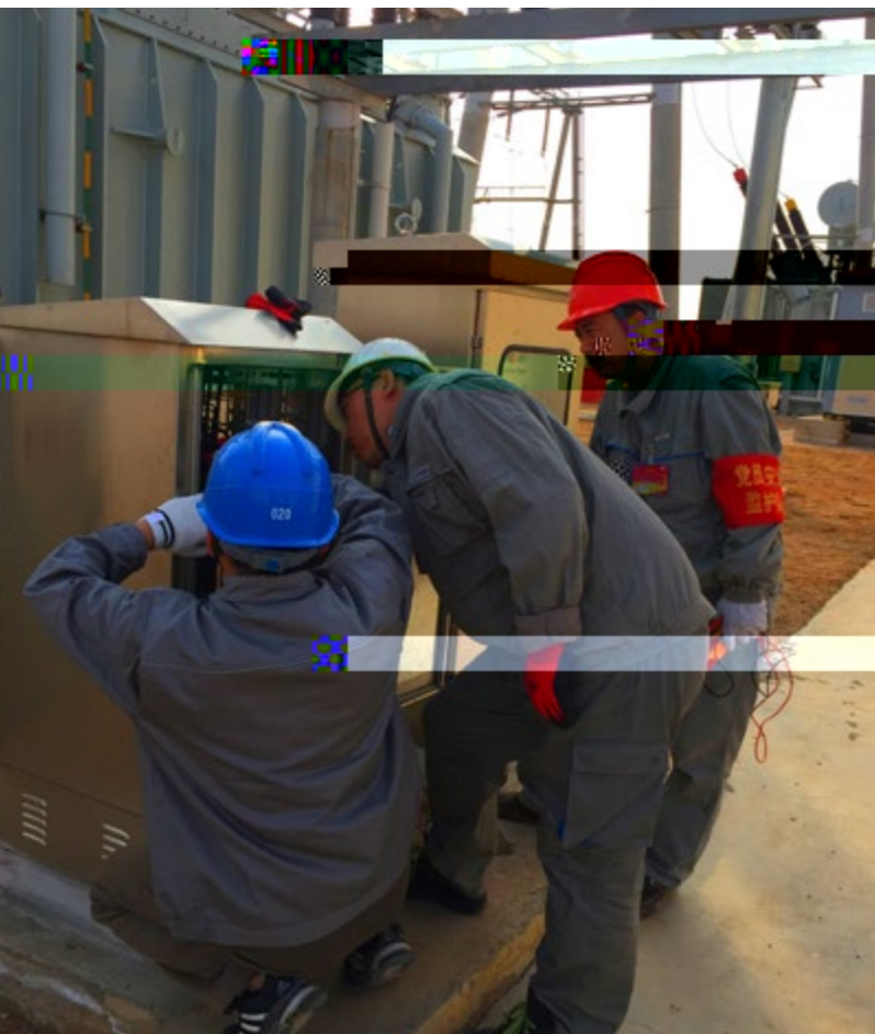
Longyuan Neimenggu Company enhance their equipment defect treatment as shown in the picture of Saiwusu wind farm booster station.
