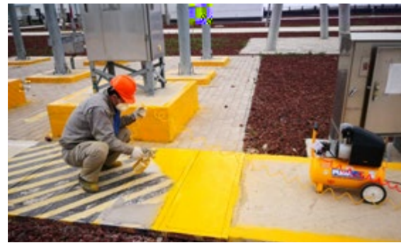
On July 12, 2018, the maintenance personnel of Xinghe Wind Farm of Longyuan Inner Mongolia Company carried out the warning and marking paint for yellow and black in accordance with the requirements of safety and civilized standardization.
