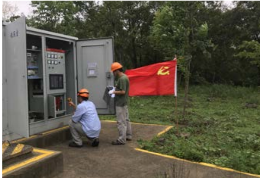
On the eve of the Super Typhoon Lekima's landing, the wind farms of Longyuan Jiangsu Company carried out special inspections to investigate and eliminate hidden troubles.
